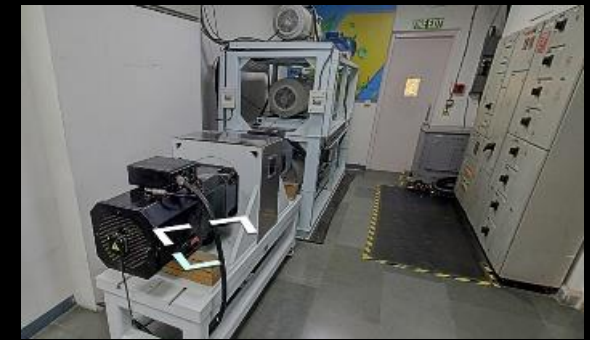
Power Electronics Lab
